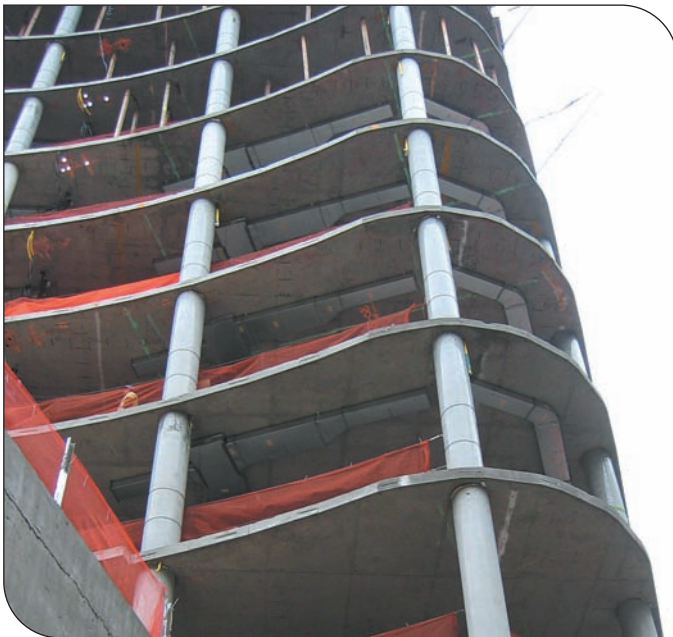
Concrete framed buildings provide thermal mass and have lower energy consumption than non-mass buildings.
