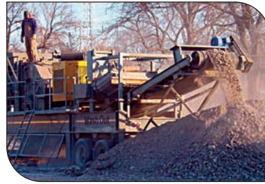
Materials and Resources Credit 2. The picture shows machinery taking portions of concrete walls, columns, and floors and crushing them to be used as fill material.
